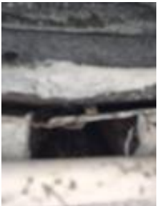
Gnagersikring - Manglende musesperre
